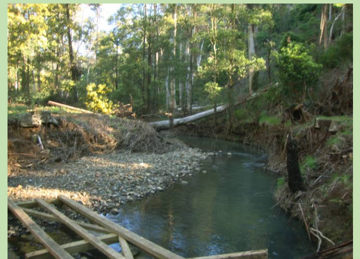
The footing to the bridge (near Billy's Weir) remain on both banks. If the bridge is to be replaced these footings could be reused.
