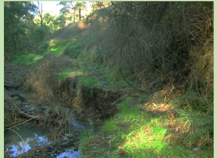
The flooded creek has underwashed the track leaving little of the original track. Blackberries and other plants will need to cut back on the bank to allow safe walking.
