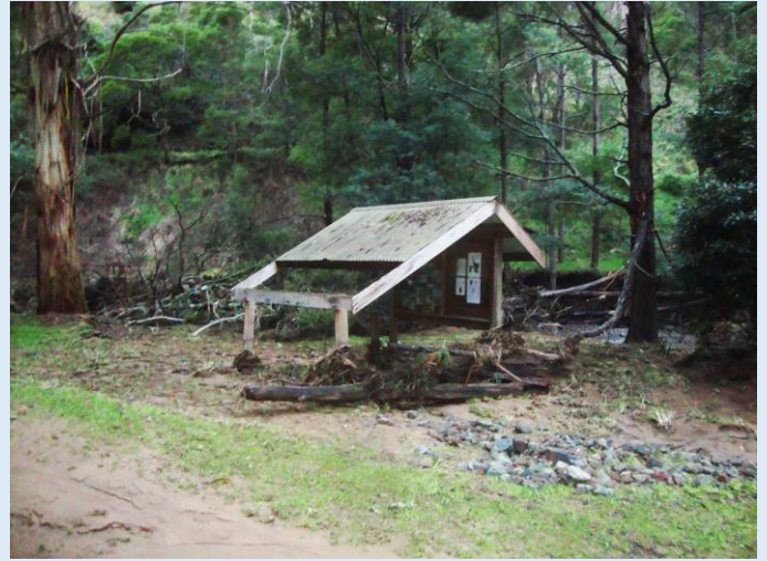
The information booth has survived but the flood water (which at its peak was at least two feet above ground level) has washed fallen limbs against the structure.
